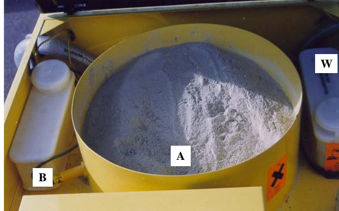
Feed System for Clay Flocculating Agent and Odor Control/Biocidal Agent
